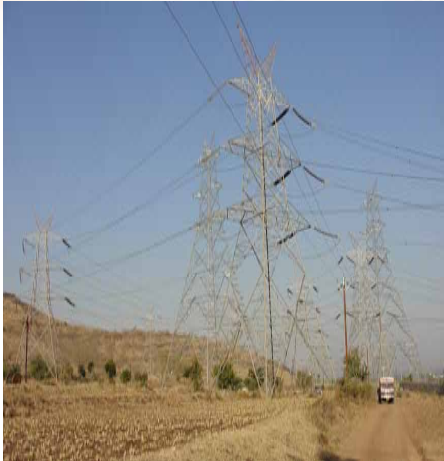
400 KV Power line crossing at Karad End
